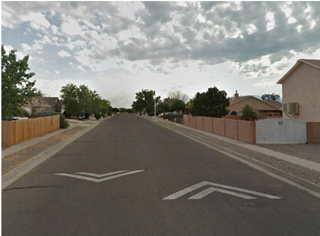
Figure 7: Tanager Drive Existing Speed Hump
